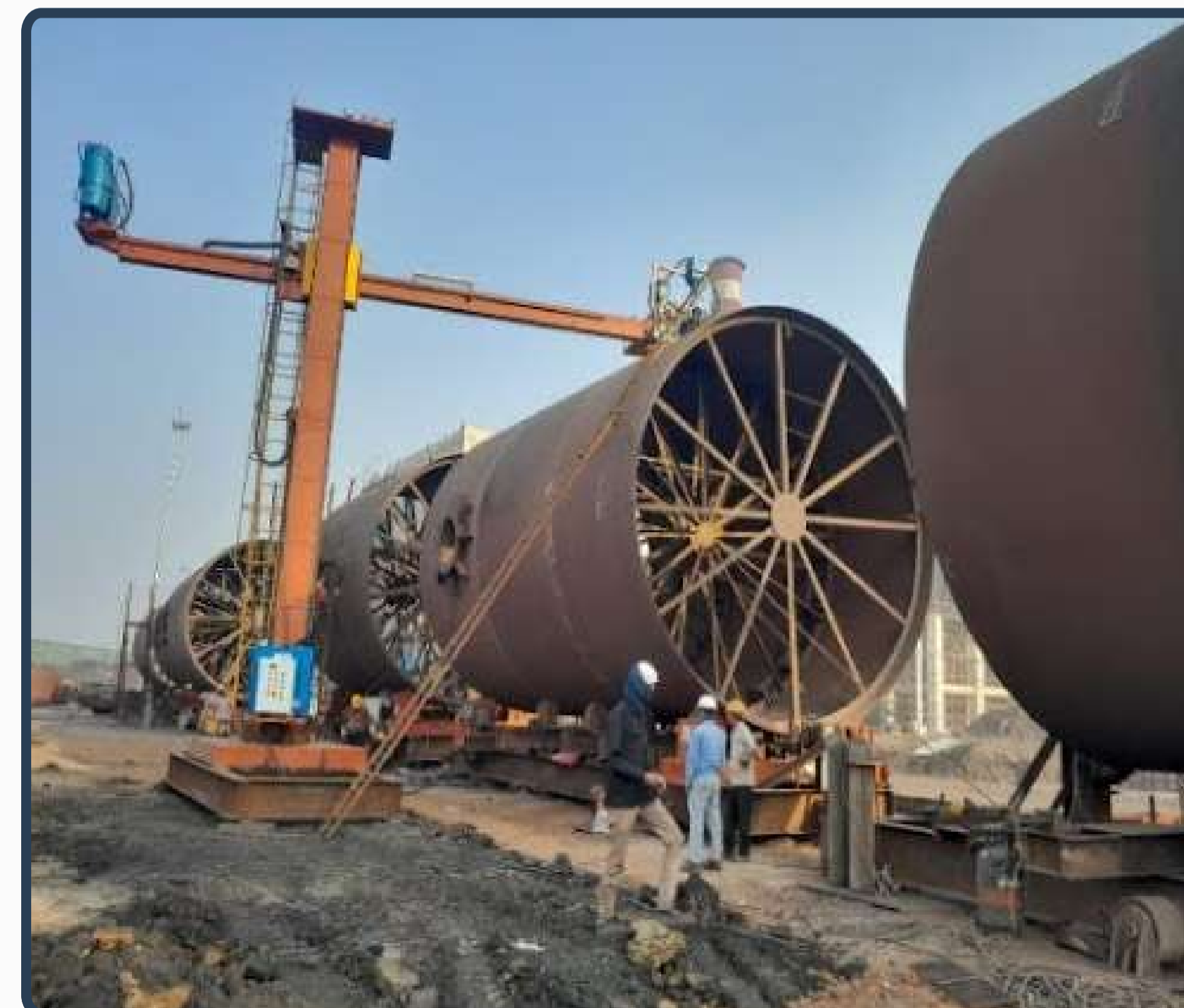
Erection of 900 TPD klin in a single day (9 hrs) at RASHMI. Single-day erection record 1060 MT at RASHMI
