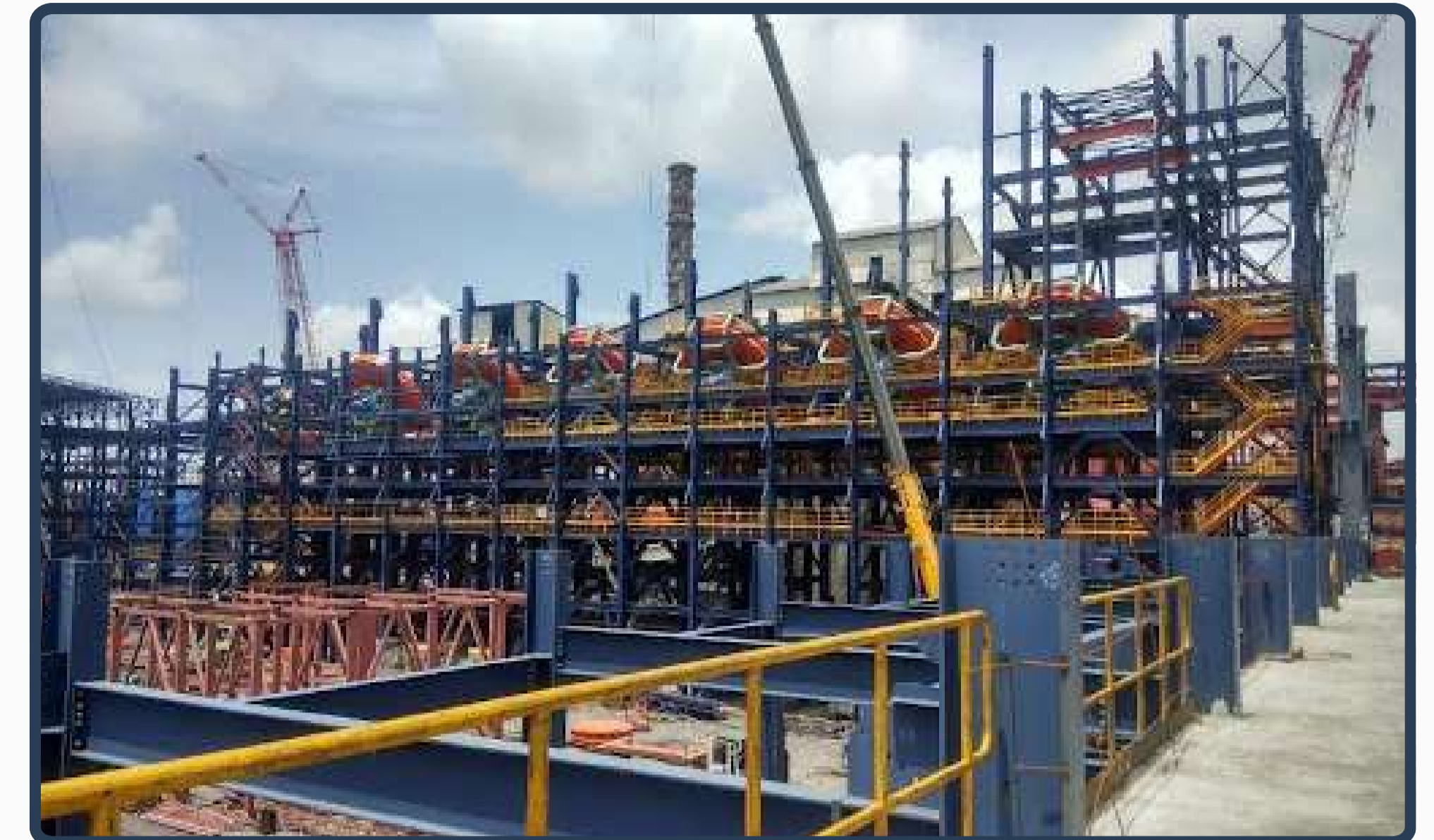
World Biggest Pellet Plant (8MTPA) For JSW DOLVI, (Supply, Erection & Commissioning -11 Months)
